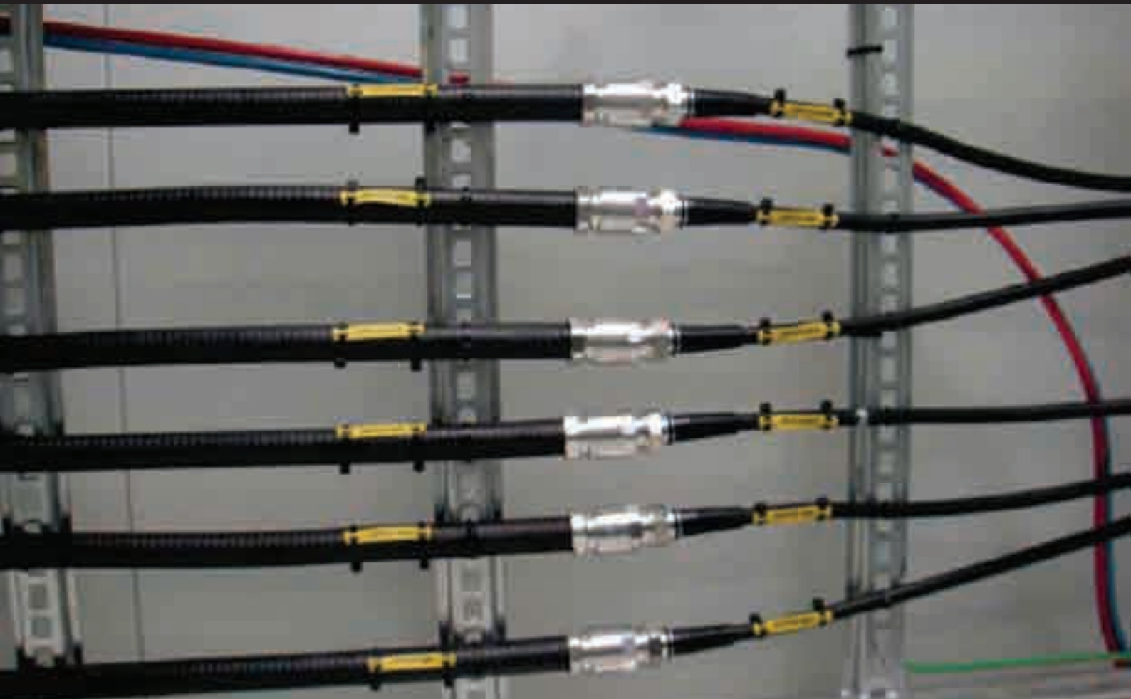
Feeder termination and labeling
