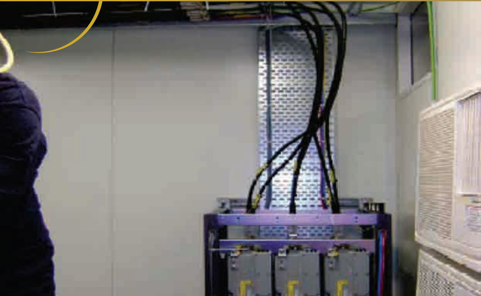
BTS installed and commissioned
